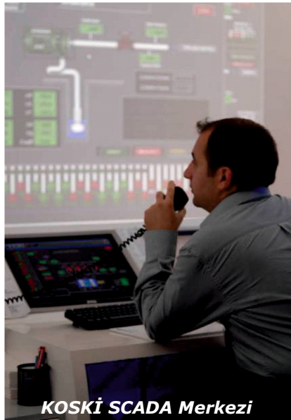
KOSKİ SCADA Server
