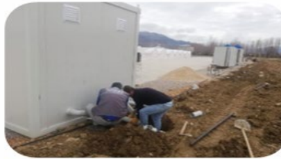
GBM (10 Bin) Su, Banyo, WC
